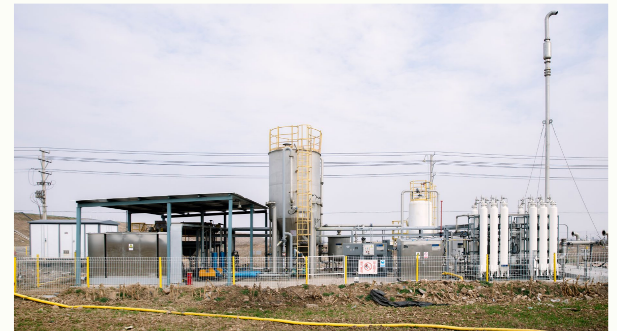
Biogas Purification System
